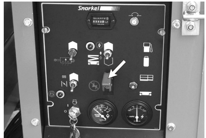
Figure 8.1 - Emergency Stop Switch at Ground Control Box
