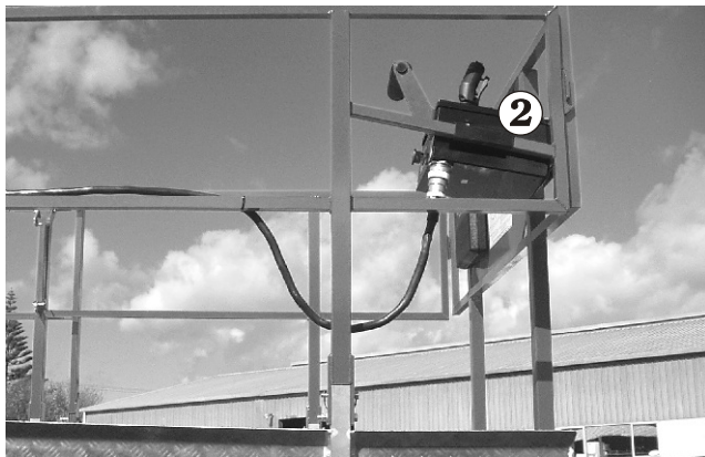
Figure 6.1.2 - Control Box Location, Platform Position
