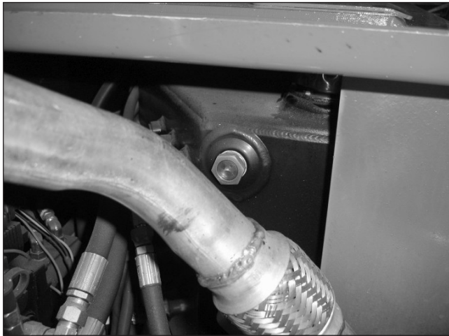
Figure 7 – Hydraulic Fluid Reservoir
