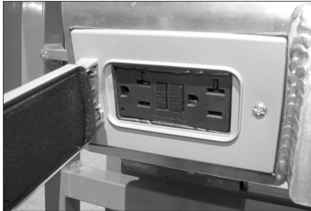
Figure 9.6 – Electrical Power Outlet
