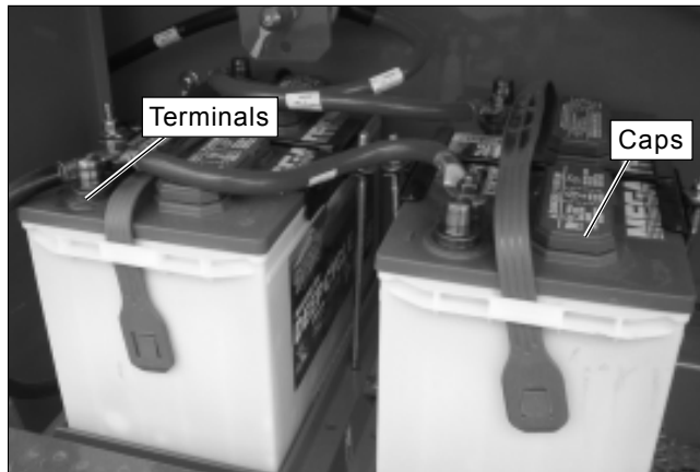
Figure 7.6 – Emergency Power Battery
