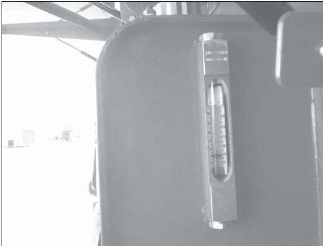
Figure 8 – Hydraulic Fluid Reservoir
